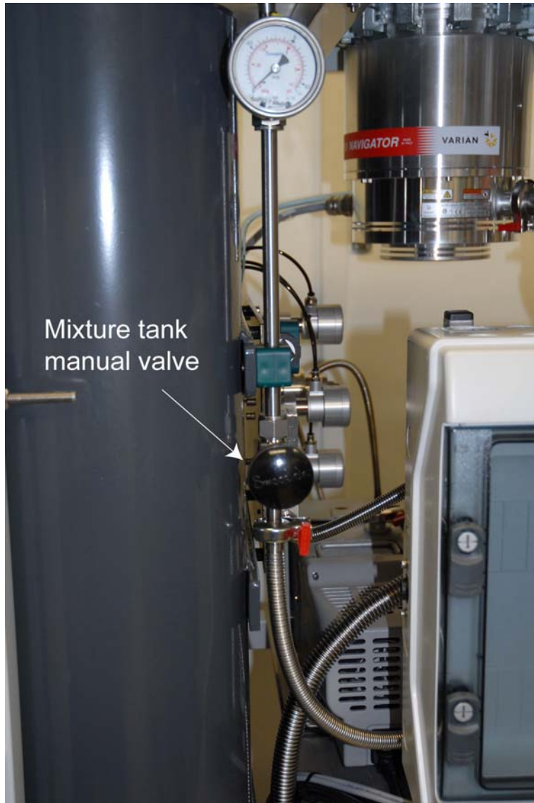
Figure 18. Mixture tank manual valve.
