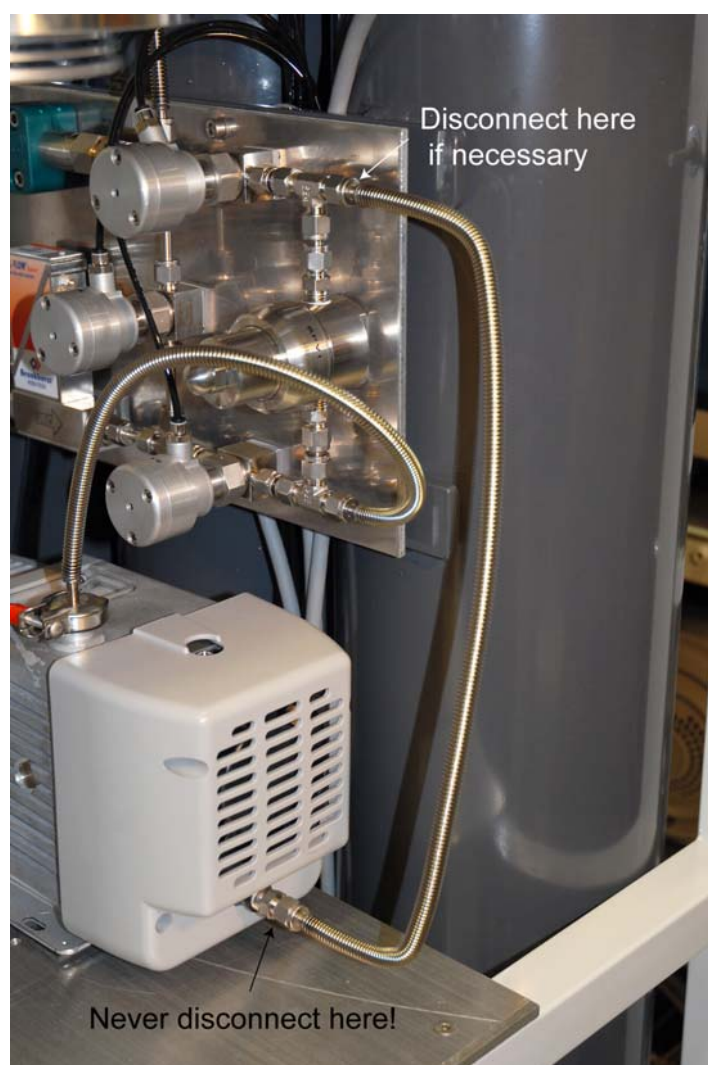
Figure 24. Compressor service warning.
